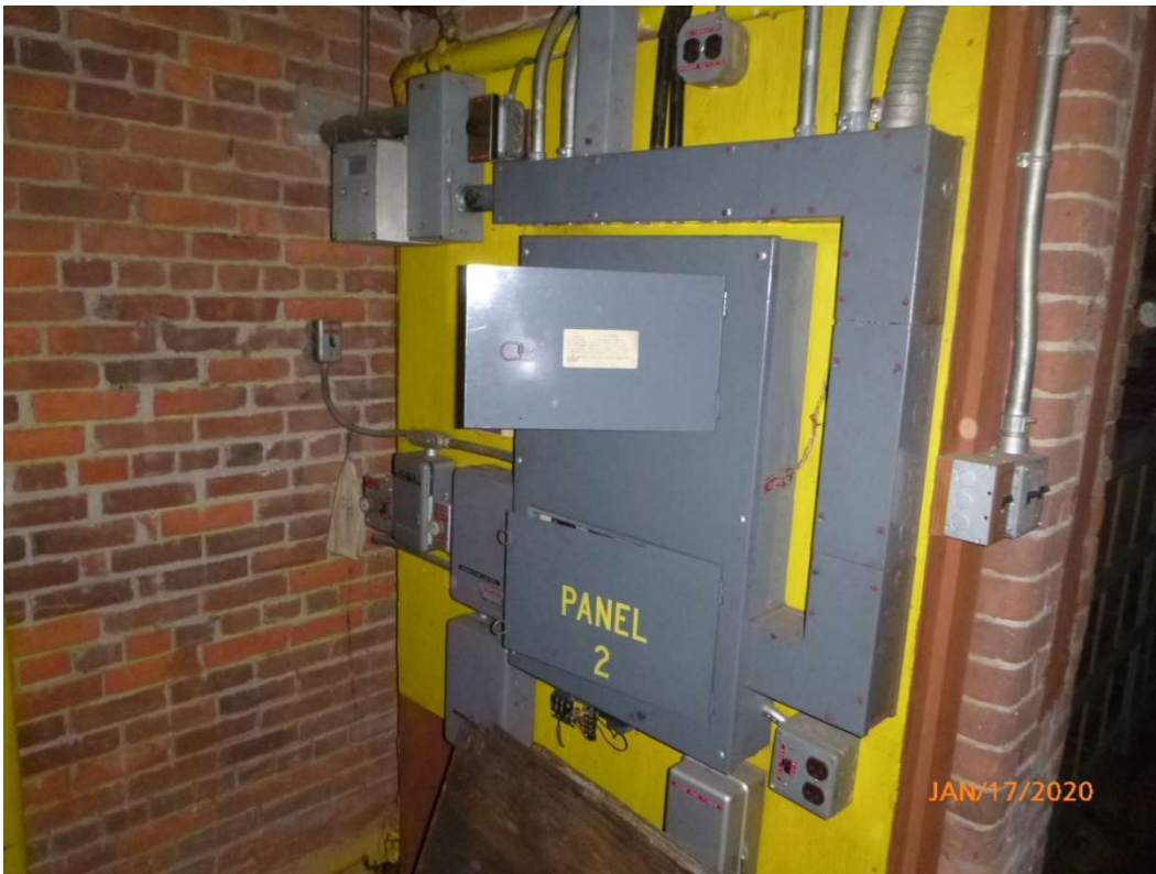
Photo 26. Electrical panel on the west side of the building in the manufacturing room.
