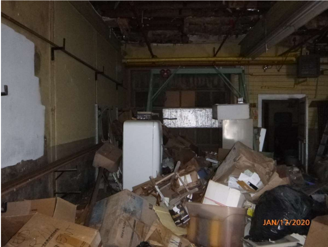
Photo 45. Storage area in the northwest corner of the building inside the backdoor.
