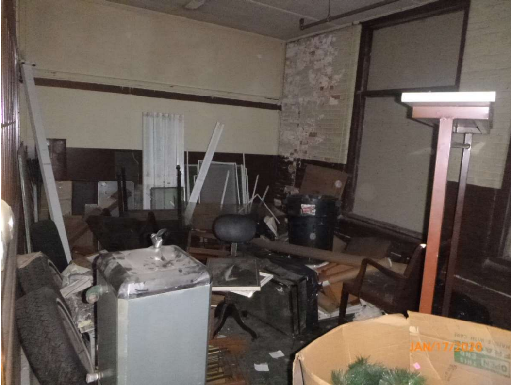
Photo 5. Inside of one of the second floor offices located on the west side of the building.
