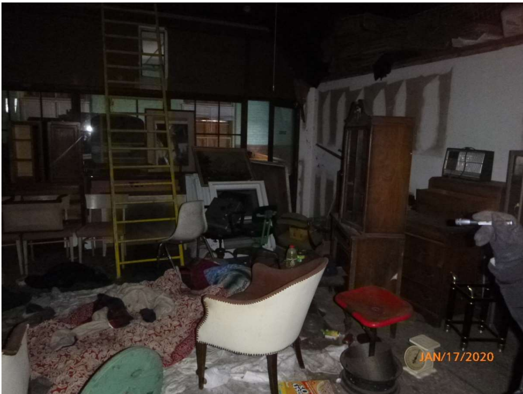
Photo 4. View of the second floor storage area looking toward the back of the building.
