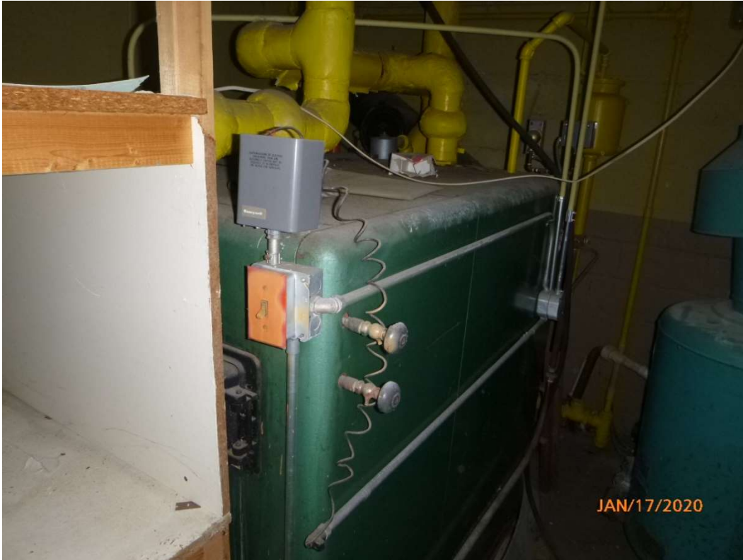
Photo 35. Boiler used to heat the building, on the west side of the building.
