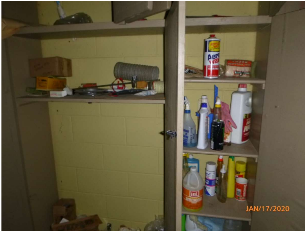
Photo 13. Cleaning supplies storage in the sprinkler system room.
