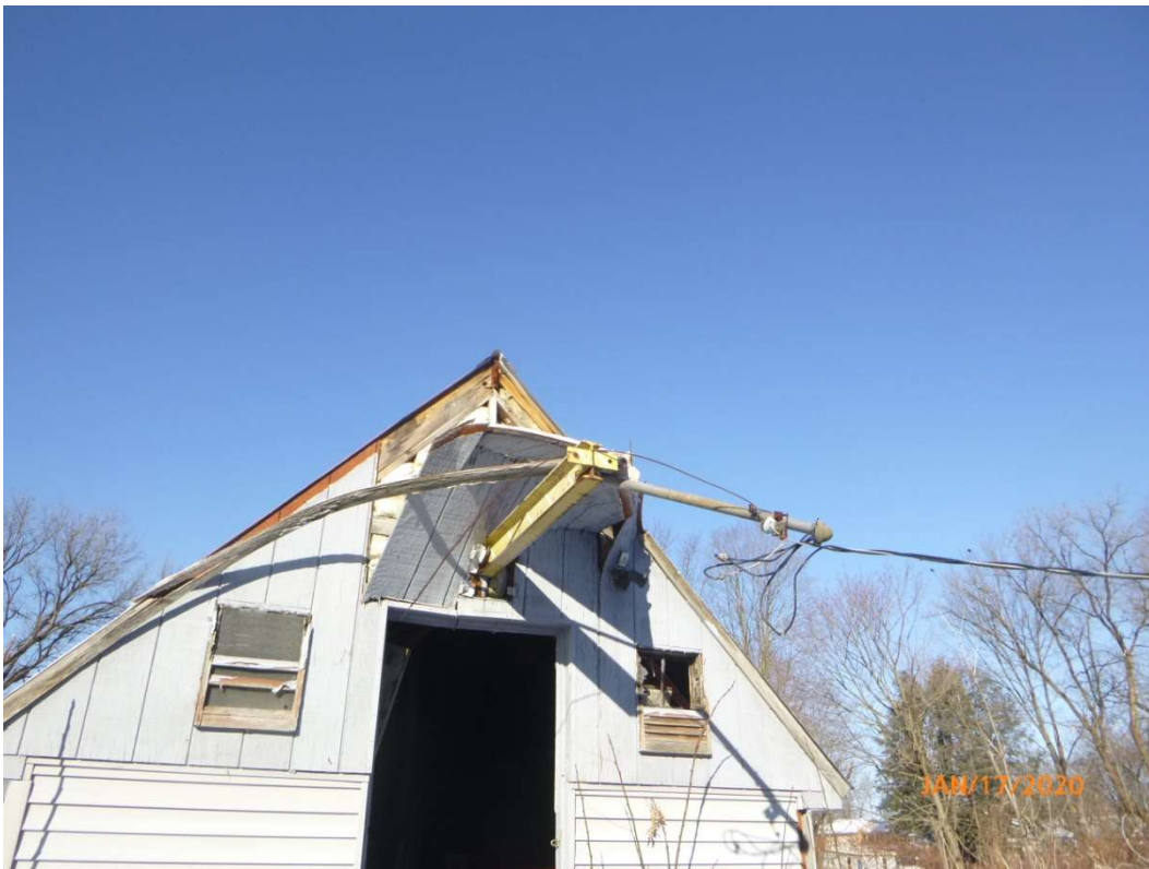
Photo 52. Electrical lines going to the outbuilding on the property.
