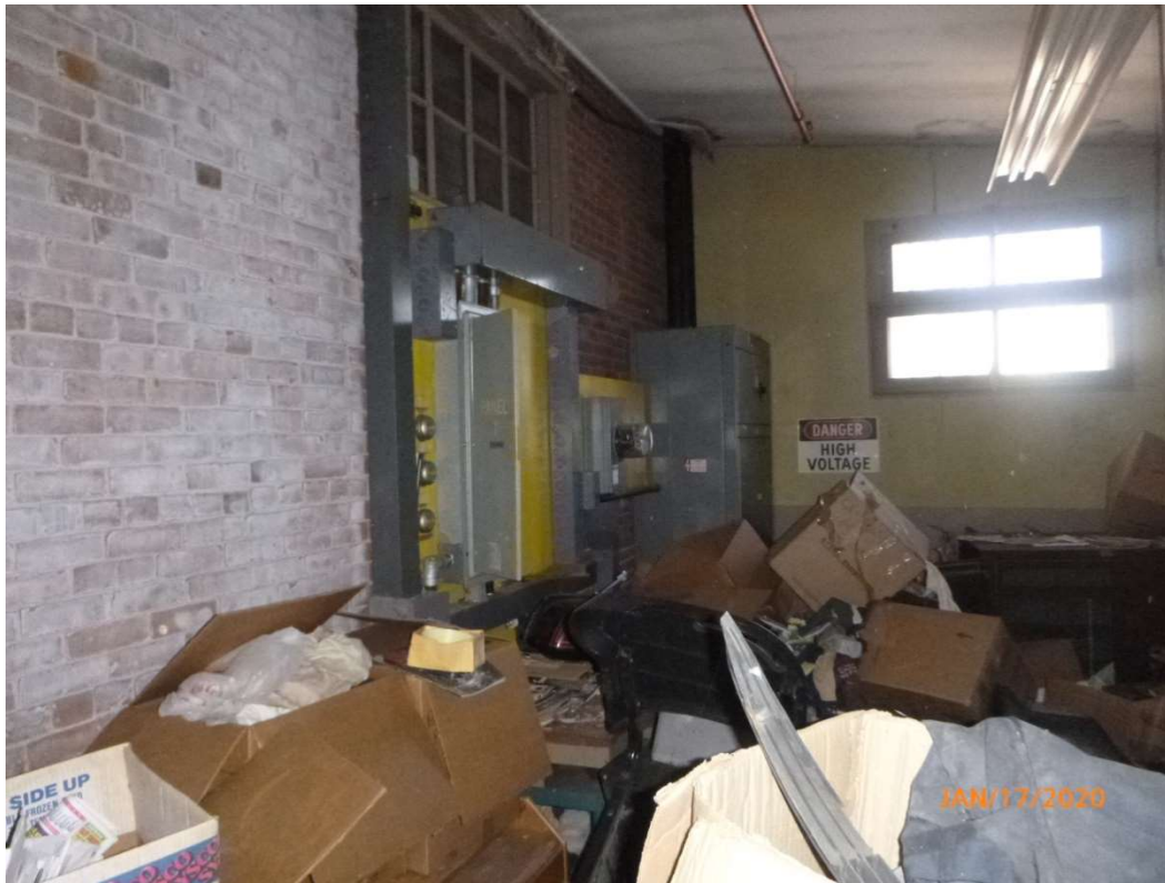
Photo 17. Breaker panels on the east side of the building.
