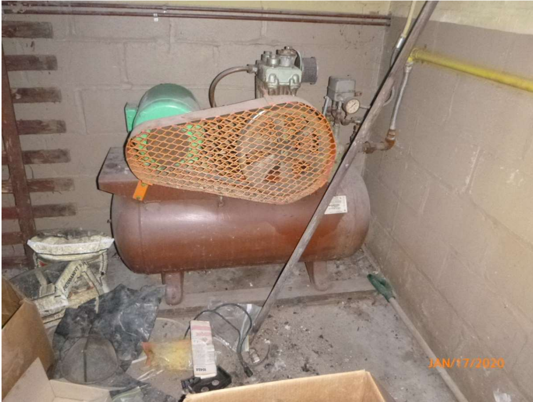
Photo 31. Air compressor in the boiler room along the west wall of the building.
