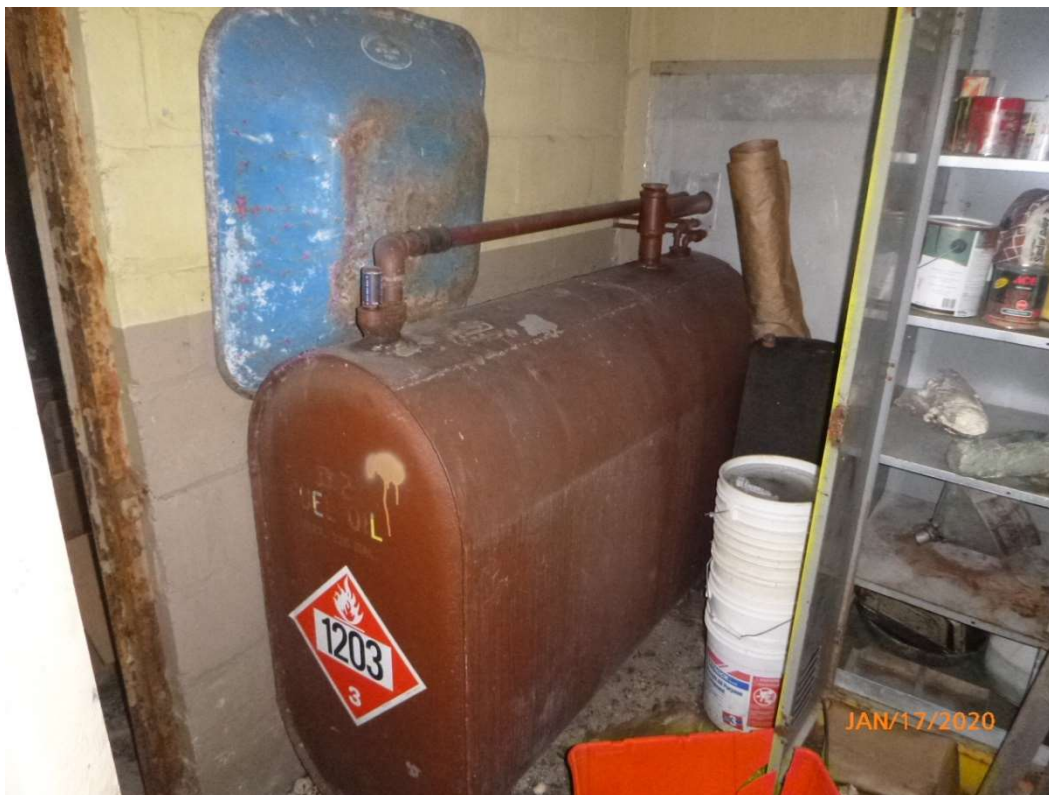
Photo 30. 225 gallon fuel oil tank outside of the boiler room.
