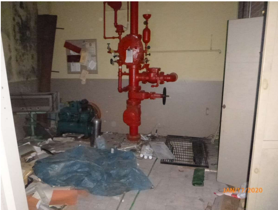
Photo 10. Fire sprinkler system located in the northwest corner of the building.
