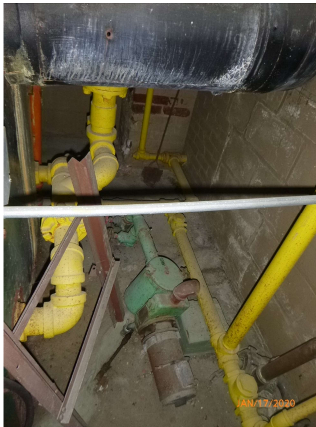
Photo 36. Back of the boiler.
