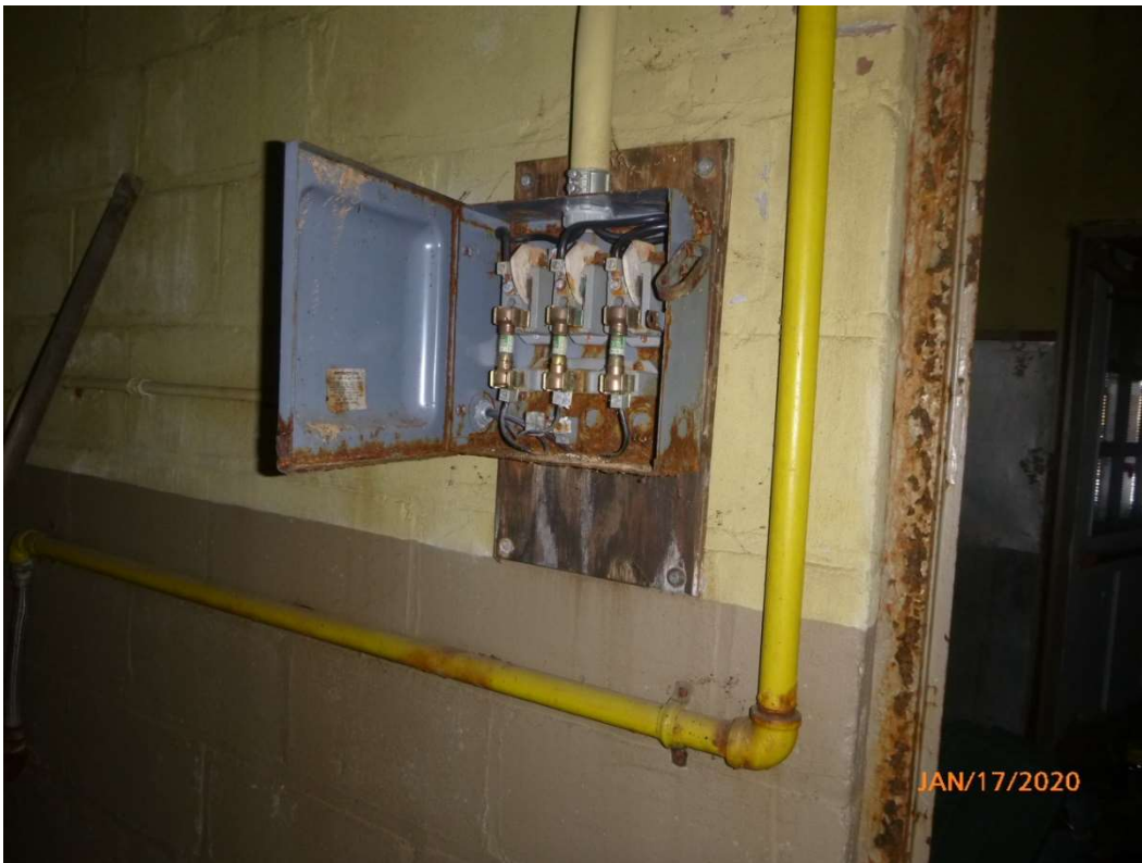
Photo 32. Electrical unit within the boiler room.
