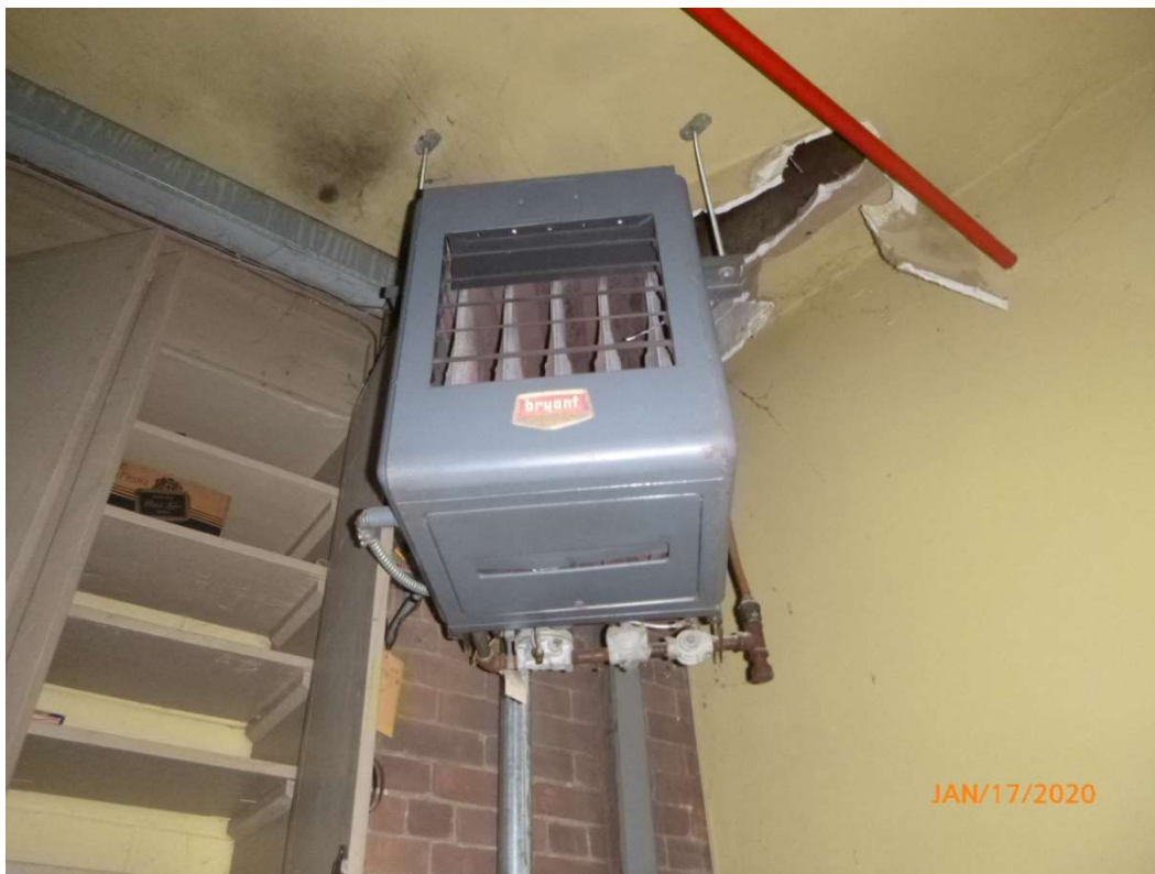
Photo 14. Bryant heating system in the sprinkler system room.
