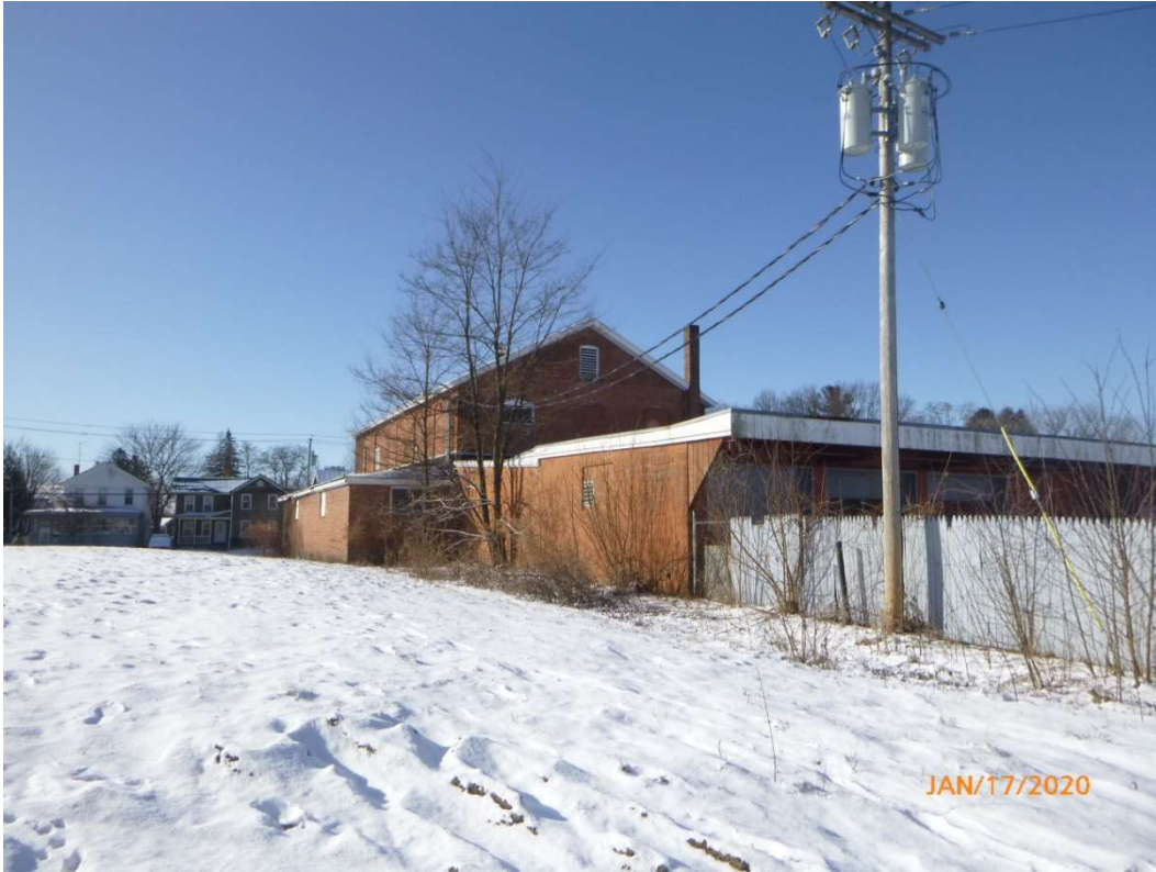
Photo 57. View of the east side of the building and transformers.
