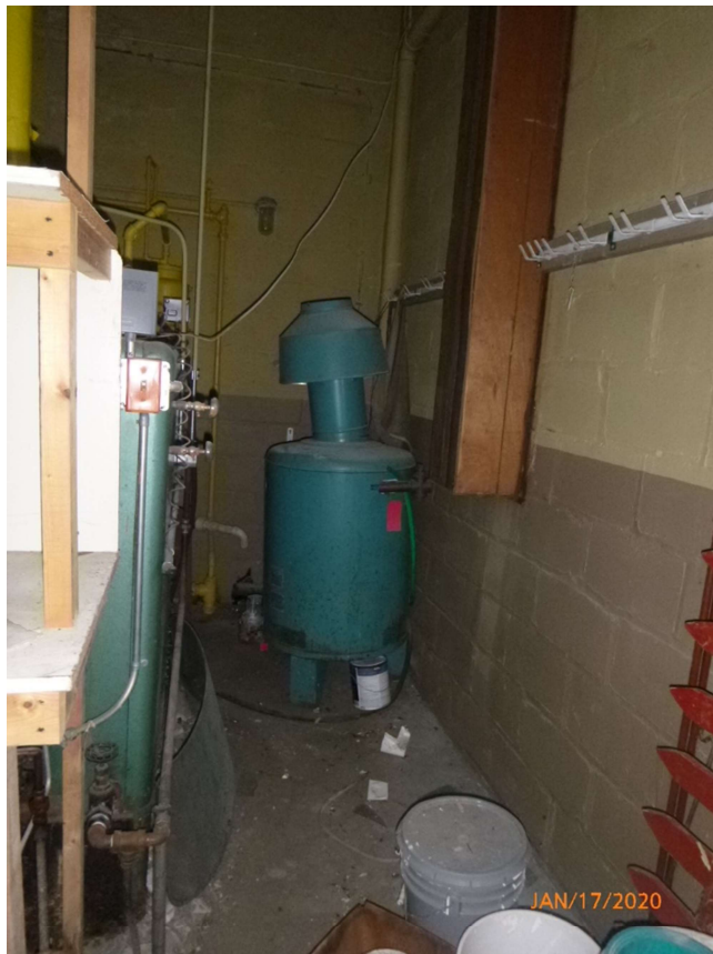
Photo 34. Area next to the boiler.
