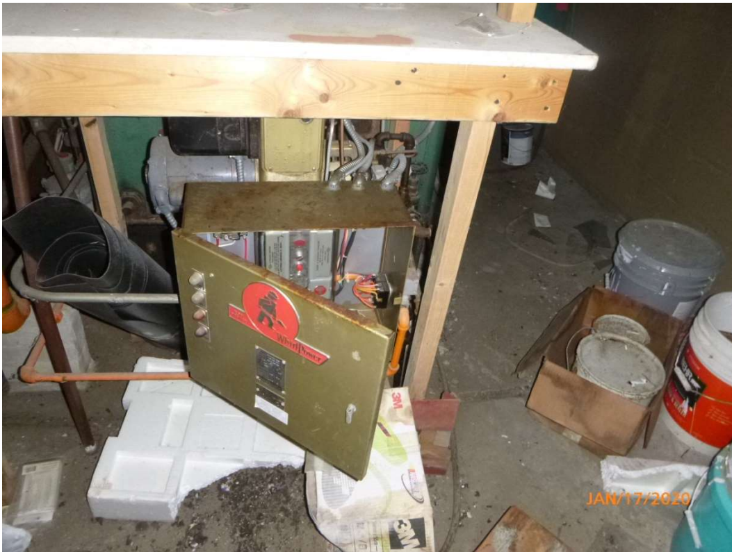
Photo 33. Electrical panel for the Iron Fireman WhirlPower boiler.
