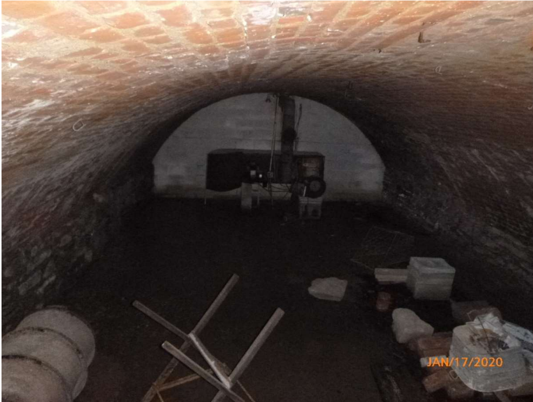
Photo 55. Equipment in the basement of the outbuilding.
