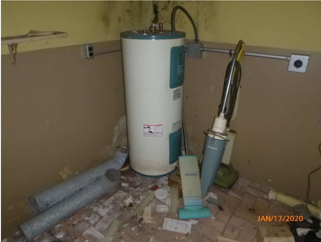
Photo 11. Hot water heater located in the sprinkler system room.
