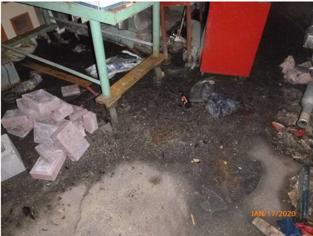
Photo 28. Floor of the hall outside of the boiler room on the west side of the building. Petroleum residue and metal filings visible.
