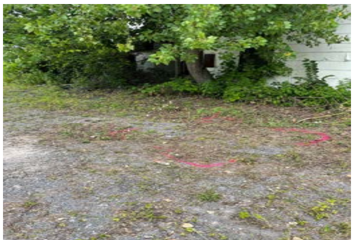
View of parabolic anomaly at the rear of the Residential building identified during GPR facing northwest.
