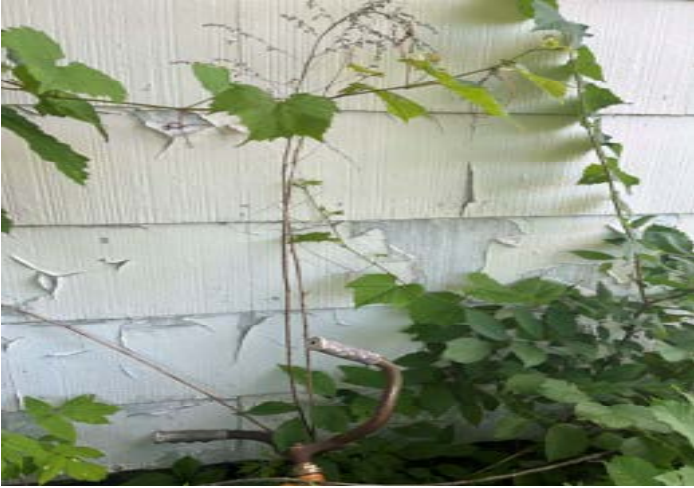
View of suspected lead paint peeling from the rear of the Residential building facing south.
