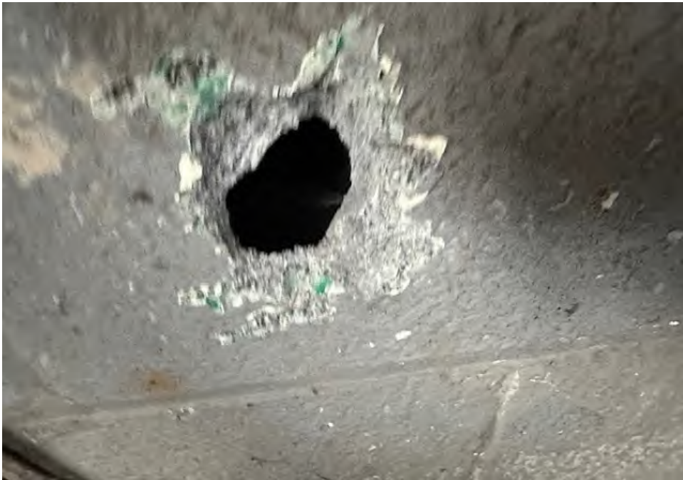
Garage wall - no vermiculite
