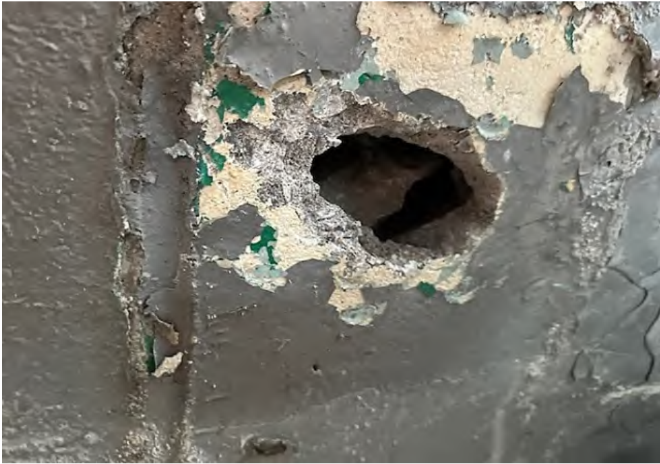
Garage wall - no vermiculite
