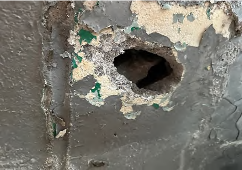
Garage wall - no vermiculite
