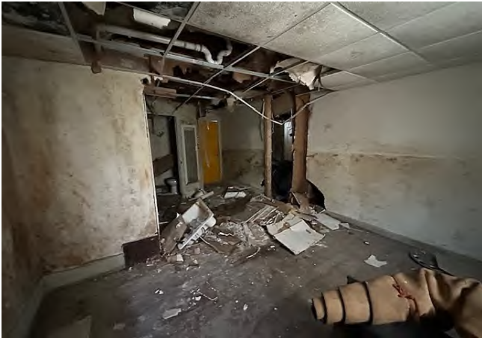
room #1 - debris pile
