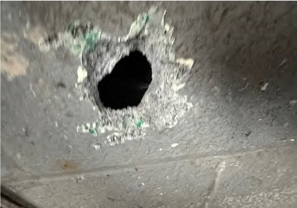
Garage wall - no vermiculite
