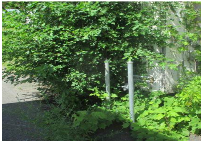
View of natural gas utility connection adjacent to residential dwelling.
