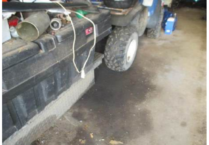
View of oil staining inside garage of Commercial building.
