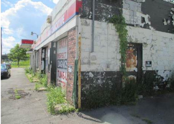
View of suspected fill pipe located on northwestern side of servicing garage.
