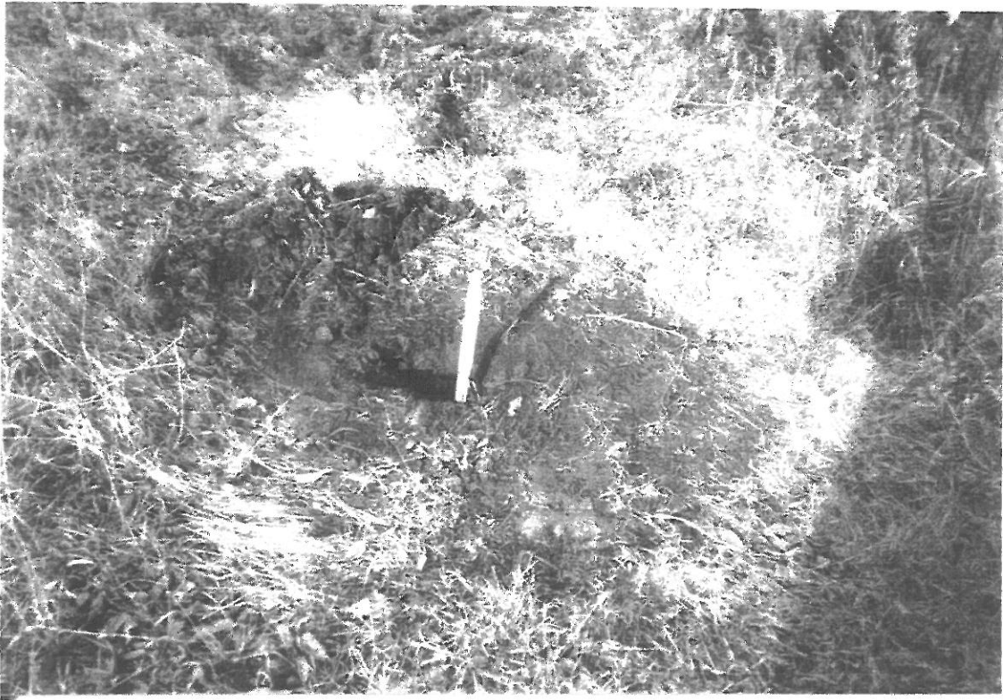
Typical Temporary Well Installation – MW1
